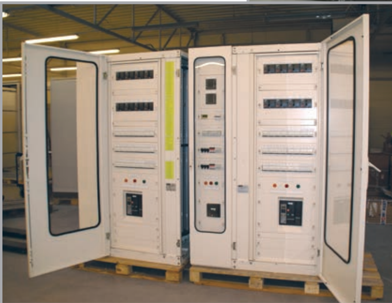
LV auxiliary systems panel, Kazakhstan
