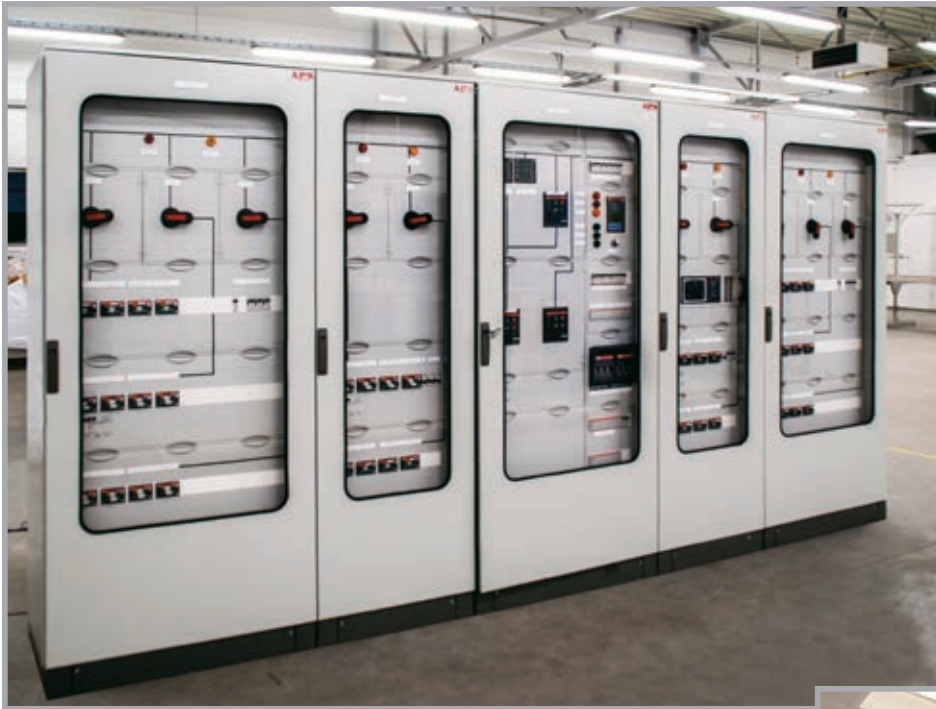
LV auxiliary systems panel of 110 kV distribution station, Russia
