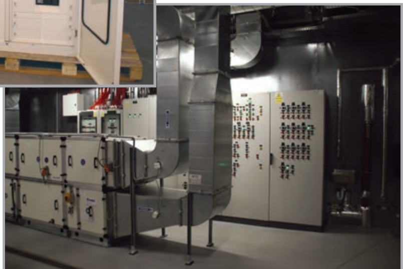
Ventilation systems control panel, line II of Warsaw Metro
